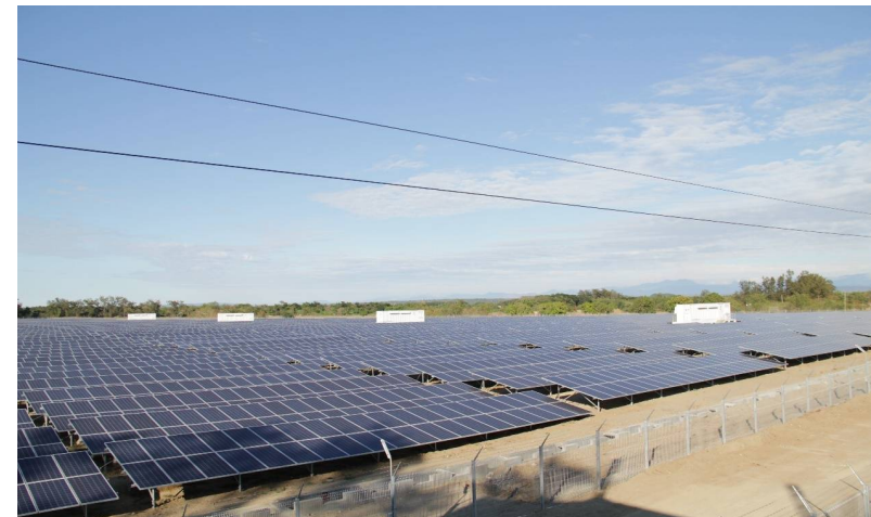
20.1 MW Currimao Solar Farm
