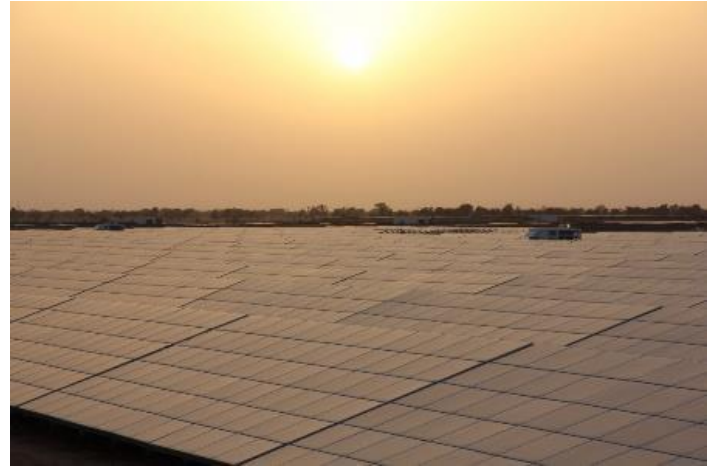
15.6 MW solar farm Pokara, Rajasthan, India
