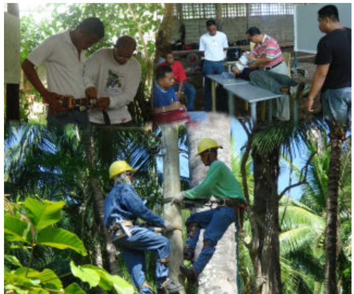
(Clockwise) Engr. Romulo Garduque ( 2nd from right) and Greg Arquero (in striped shirt) instruct trainees from ROMELCO on safety techniques during the Basic Linemen Training Course in Romblon from May 22-June 16, 2007. Bottom picture shows ROMELCO trainees during the Pole Climbing Exercise.
